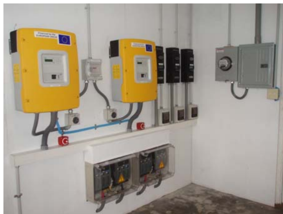
Ebon School Control Room
